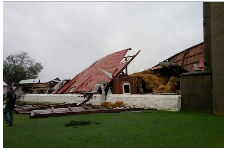
Barn damage caused by tornado in Marquette County on August 28, 2018. Source
